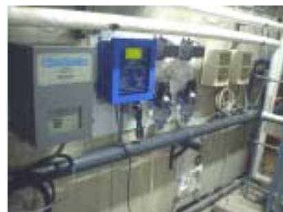
Clormatic® and Acu-Trol Installation (Above)
